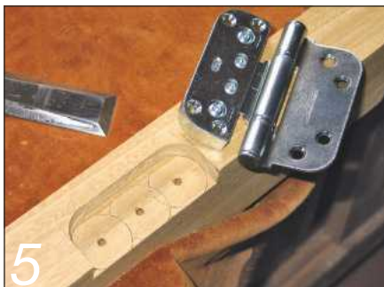
5 The hinge recesses in the door stiles are trimmed and the hinges fitted
