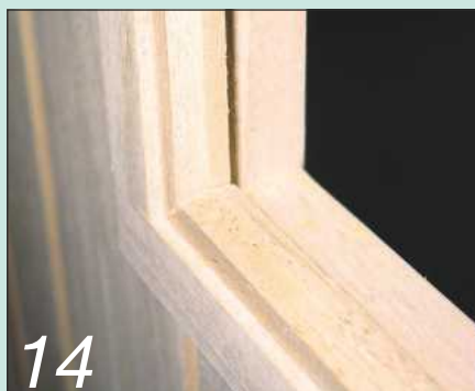
A bevelled bead finishes the glazing frame, ready for the sealed units
