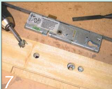
7 Holes then have to be drilled in the lock stile for the lock and handle
