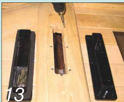
The middle door rails have an opening to accept the two-part letter box
